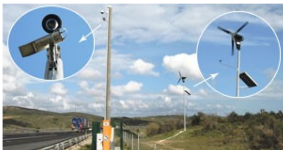
Figure 3. Highway under video monitoring
