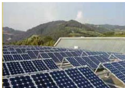
Fig. 4(2) Images installation of PV systems in Mediterranean
